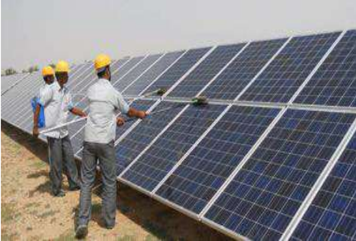
Figure 1.1 clean PV array module
